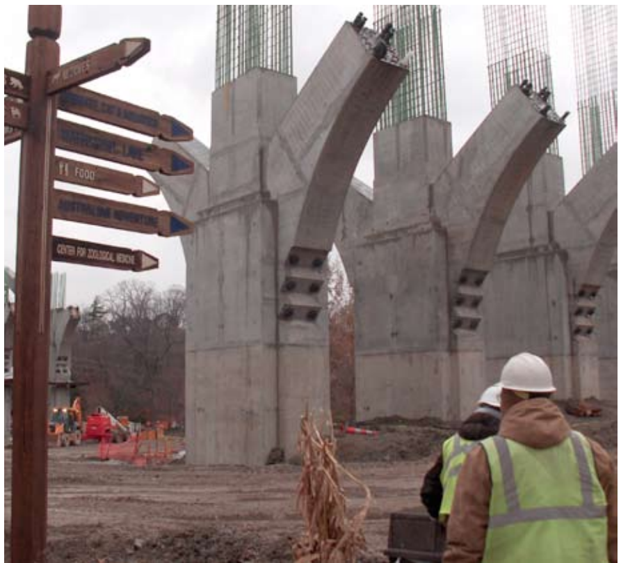
Thrust blocks located within the Cleveland Metroparks zoo. Photo: Ohio Department of Transportation.
